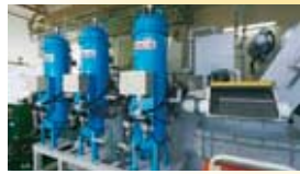
Energy and Resource-saving systems
